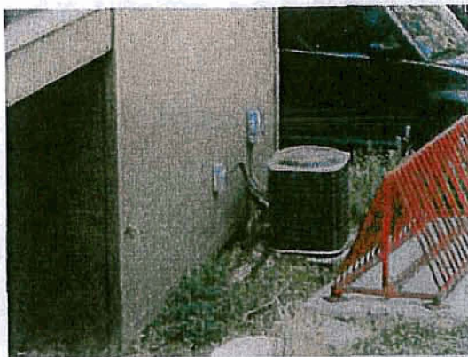
This HVAC system at 271 Center Street is situated in an inconspicuous area on the rear elevation.
