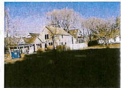
New house under construction. (Photo courtesy of Utah State Historic Preservation Office.)
