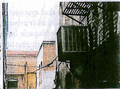
Heating and cooling units should be located at rear elevations such as shown here or on rooftop areas not visible from the street.
