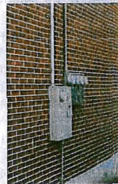
Meters at 39 North I Street are correctly placed on a non-primary elevation.
