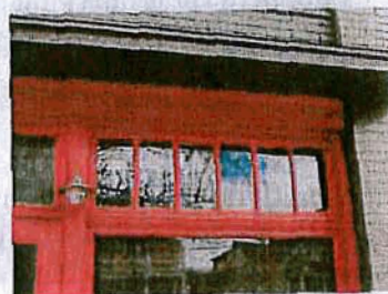
Original transoms enhance historic character and are important elements of commercial storefronts.
