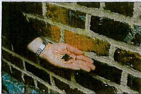
which leads to cracking and spalling.
