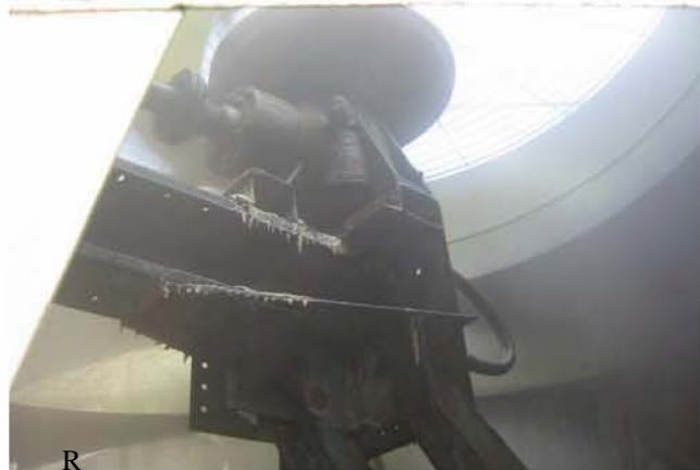
rust and corrosion are destroying the cooling tower.
