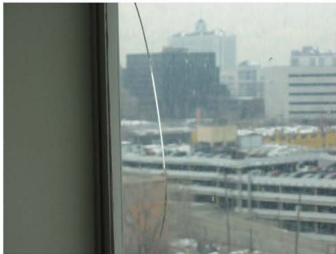
Cracked windows are not regularly replaced
