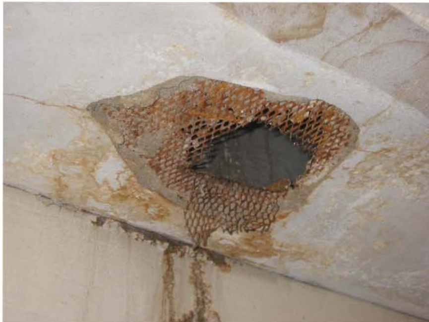
Leaking water in ceiling from water line break caused damage.
